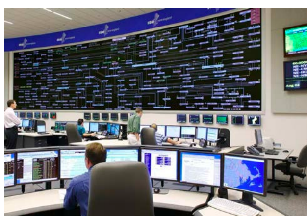
Power grid control center
